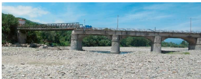
Fig. 6. The temporary Bailey bridge after the collapse of the two arches (2012)
