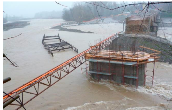
Fig. 12. Flooding during temporary phase of erections
