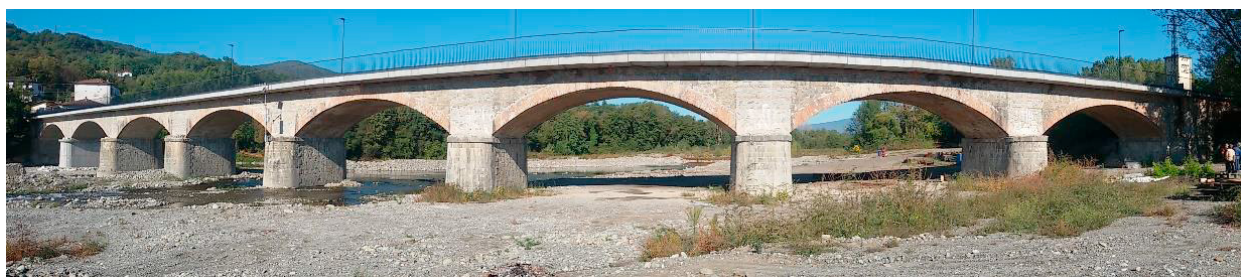
Fig. 20. A fisheye photo of the Villafranca bridge at the end of works
