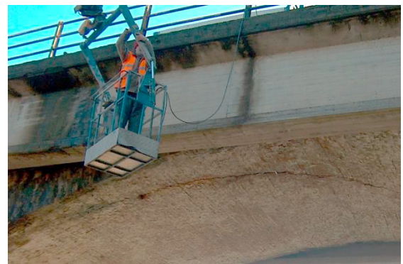
Fig. 4. Inspection of a damaged arch - monitoring phase (2010)
