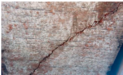
Fig. 5. Main crack on the arch (Mulazzo side 2010)
