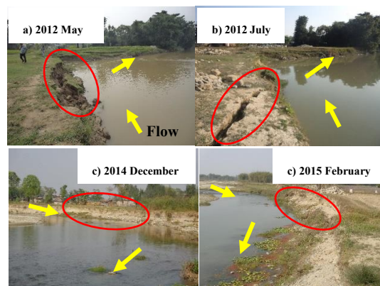
Photo 4: Bank erosion in the study reach; (a & b) Sunsari River and (c & d) Lohandra River
