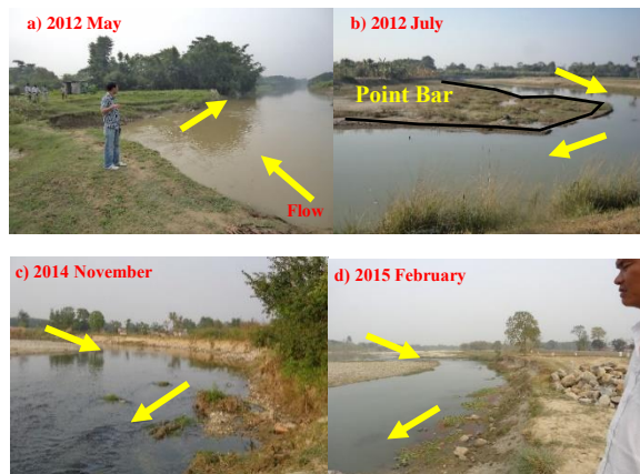
Photo 2: River Channel in the study reach; (a and b) Sunsari River, (c and d) Lohandra River
