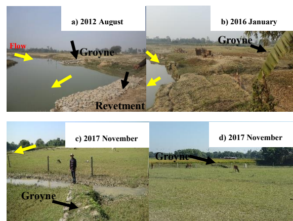
Photo 6: Implementation of Groynes for bank protection and its effect in Sunsari River.
