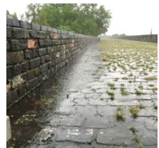
Fig. 3 Sidewalk on top of wall under rain
