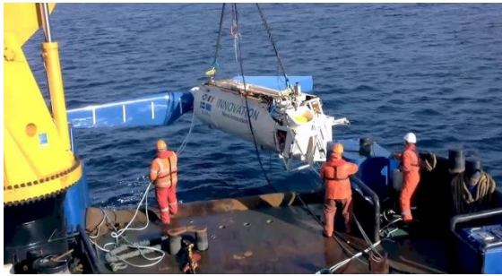
Figure 1 – Nova Innovation turbine installed at Shetland Tidal Array © Nova Innovation
