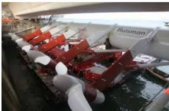
Figure 5 – Tocardo turbines at Oosterschelde. ©Tocado
