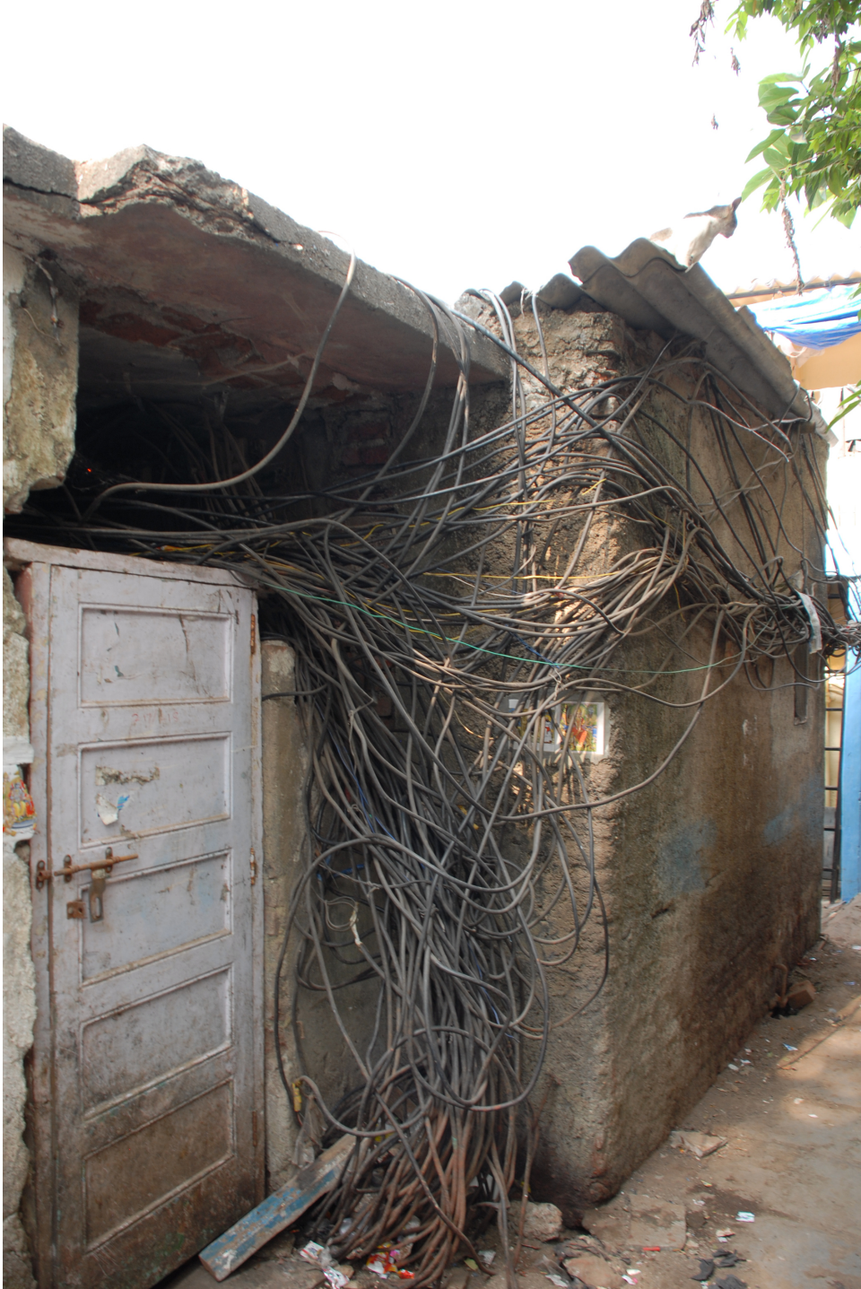
Figure 7.2 Wires leading out of an electrical substation Credit: Author
