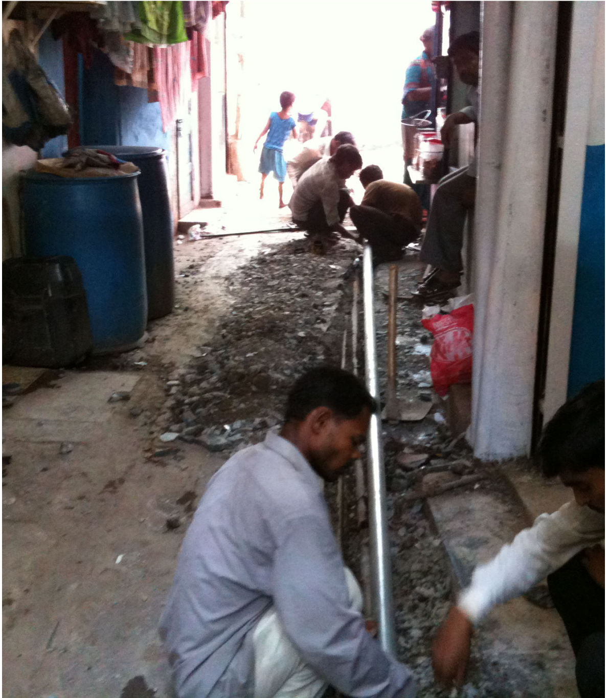
Figure 6.3 Installing a new water line for the Colaba Back Bay Association Credit: Author
