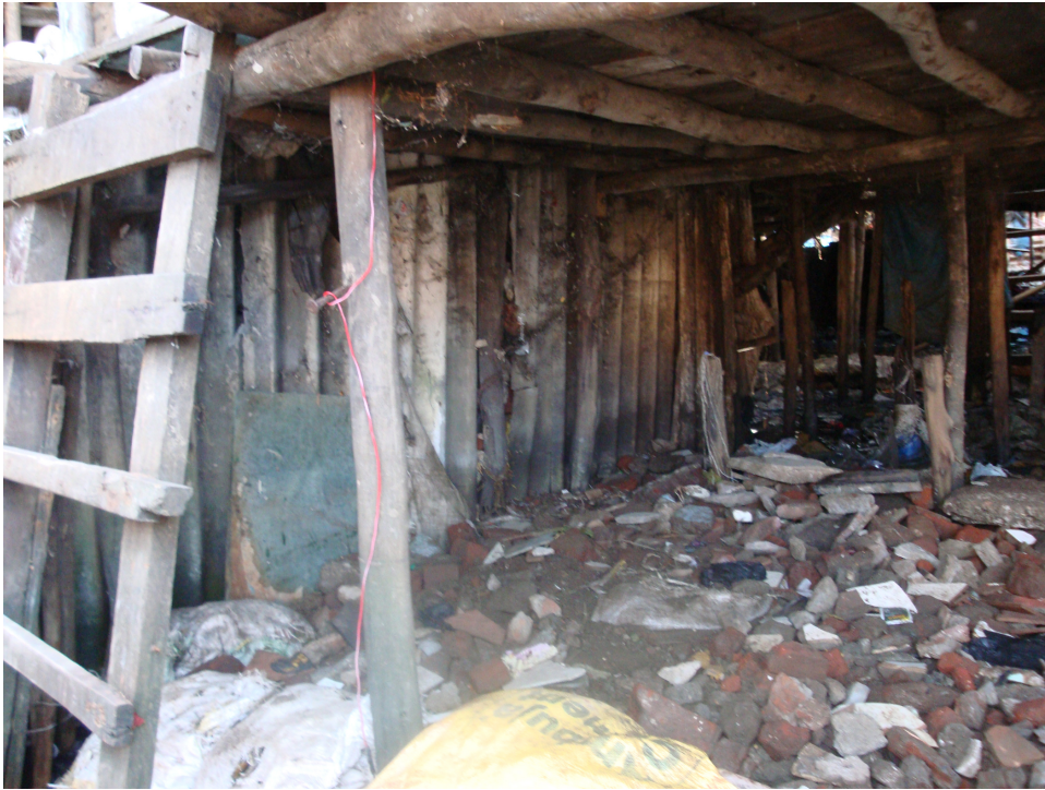
Figure 7.4 Build of refuse and debris under a hutment Credit: Author
