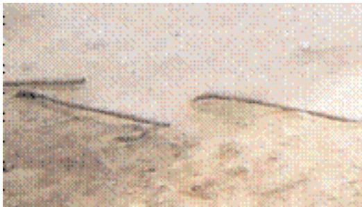
Figure 32 – Bent reinforcing steel
