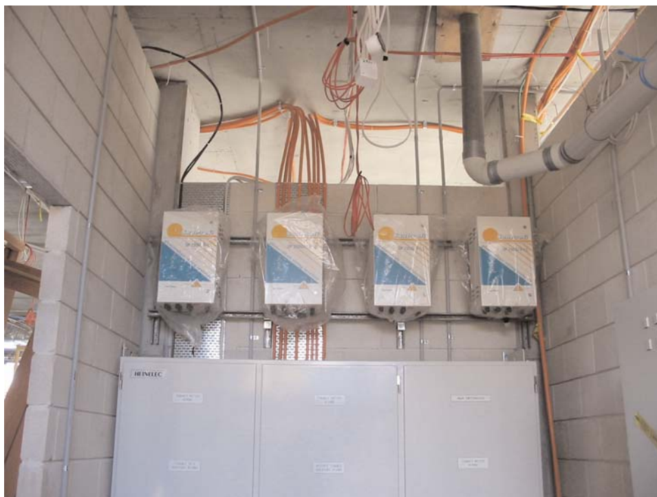
Figure 29 – inverters converting the solar energy to compatible energy to be used in the building and exported to the grid
