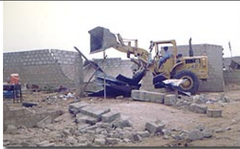
Demolition can be very brutal and mean heavy loss for informal settlement investors (Mumbai)
