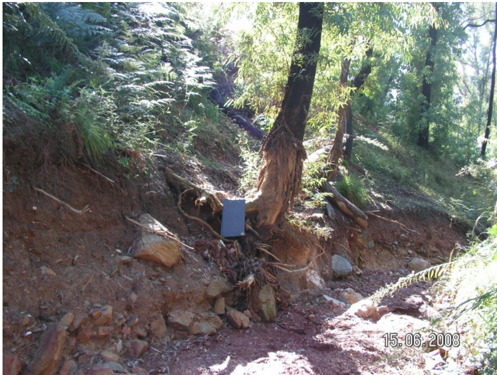
Figure 5. Scour on trees, and the channel eroded to bedrock; two key indicators of debris flow processes. Photo from Rose River headwaters in 2008.
