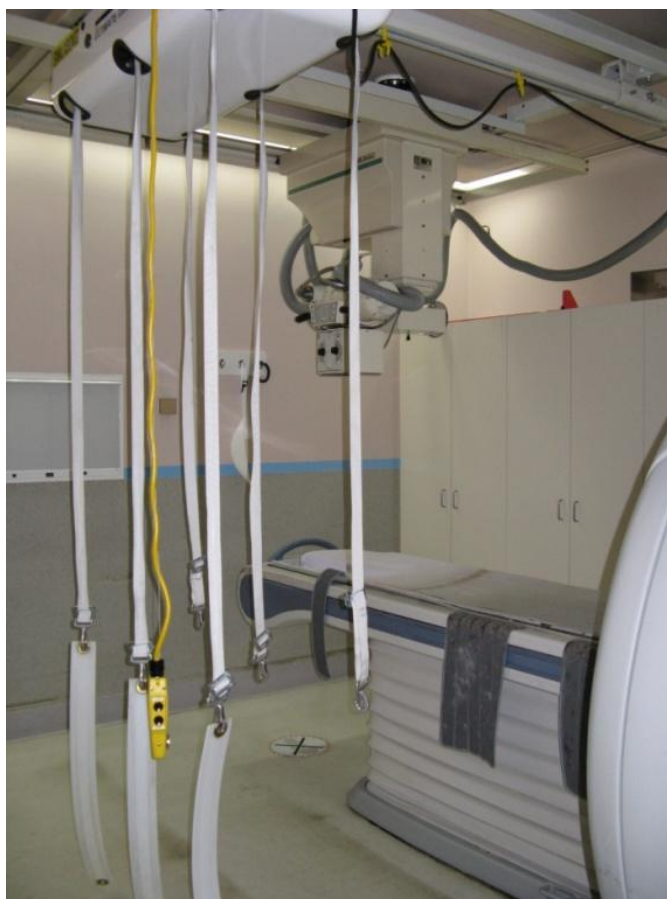
Figure 27 VIFM MDCT, heavy lifting apparatus and ceiling suspended x-ray unit
