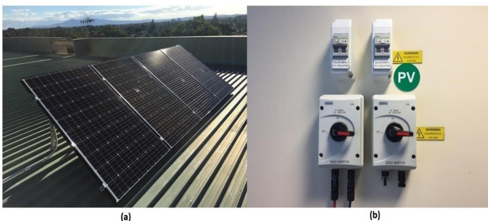
Figure 3-22: (a) 1.12 kW solar PV array installed at University of Waikato (b) Circuit breakers and isolators installed on the output side
