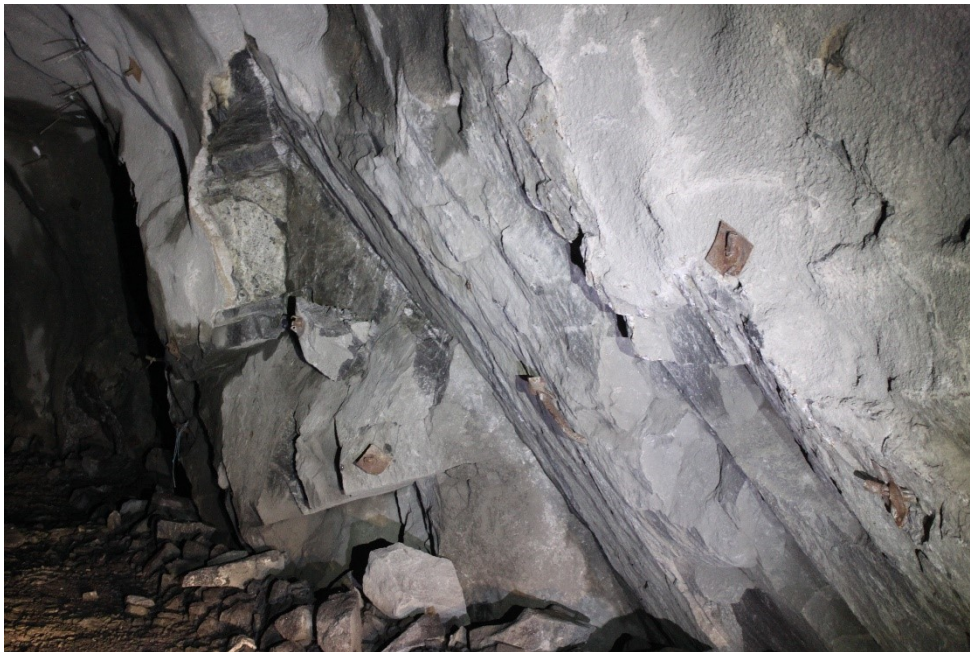
Figure 6.8: 100A22 Hangingwall present fault plane and joint structure before production commenced.
