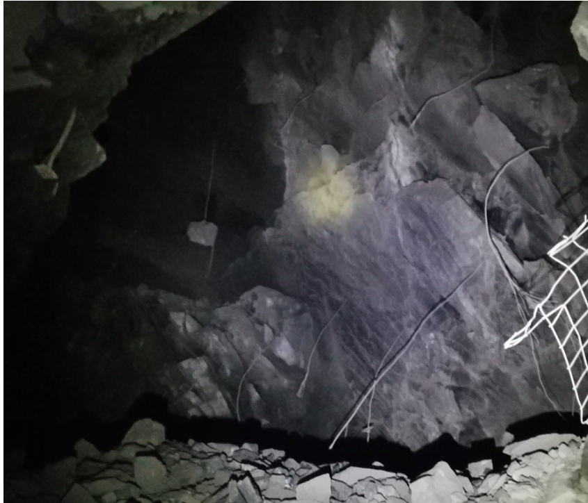
Figure 6.9: 100A22 Caving Hangingwall photographed after stope blast of rings 11-15.
