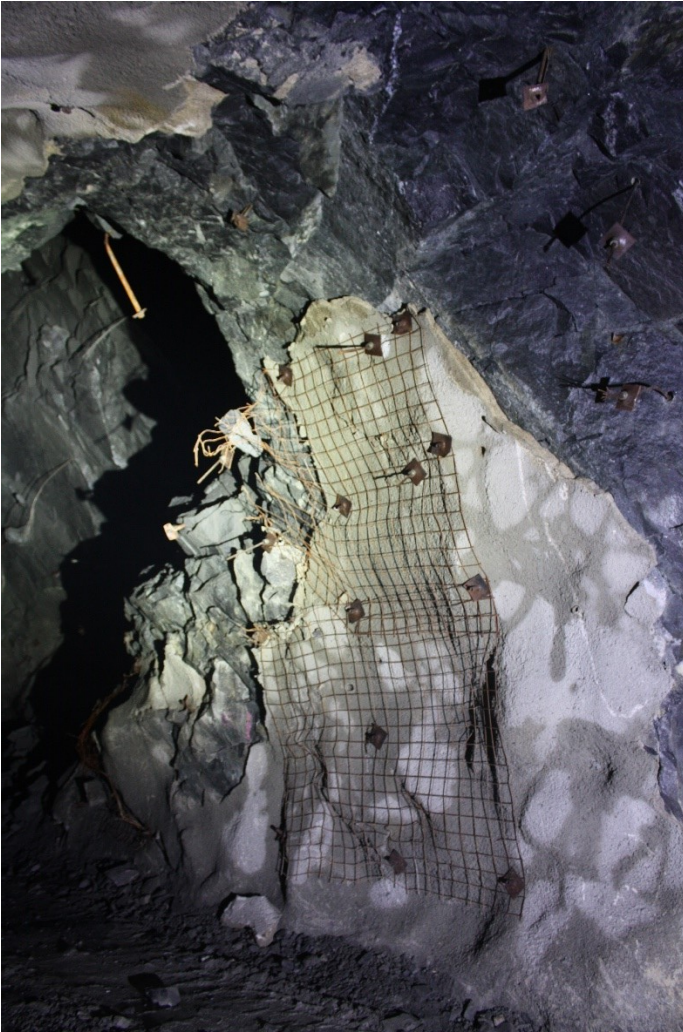
100A22 left hand side of pillar. Surprisingly intact, as part of it was designed to be mined, due to ore contact.
