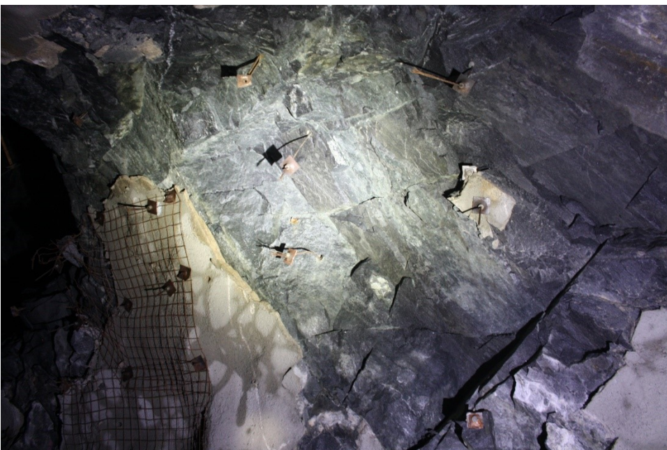
Large overview of 100A22 pillar left hand side. Installed cablebolts keeping the pillar in place.
