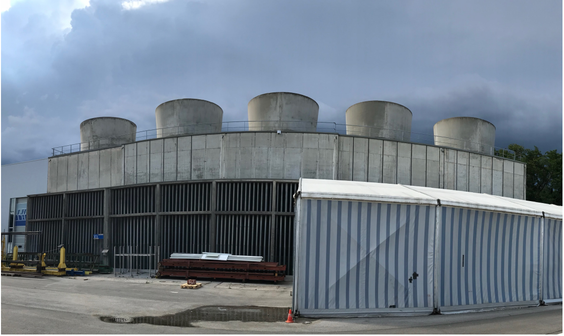
Figure 5: Cooling towers at LHC point 8 close to the Geneva Airport and the border of France and Switzerland. A tent has been blocking part of the airflow into the towers, which have increased the primary cooling water temperature during the hottest days.
