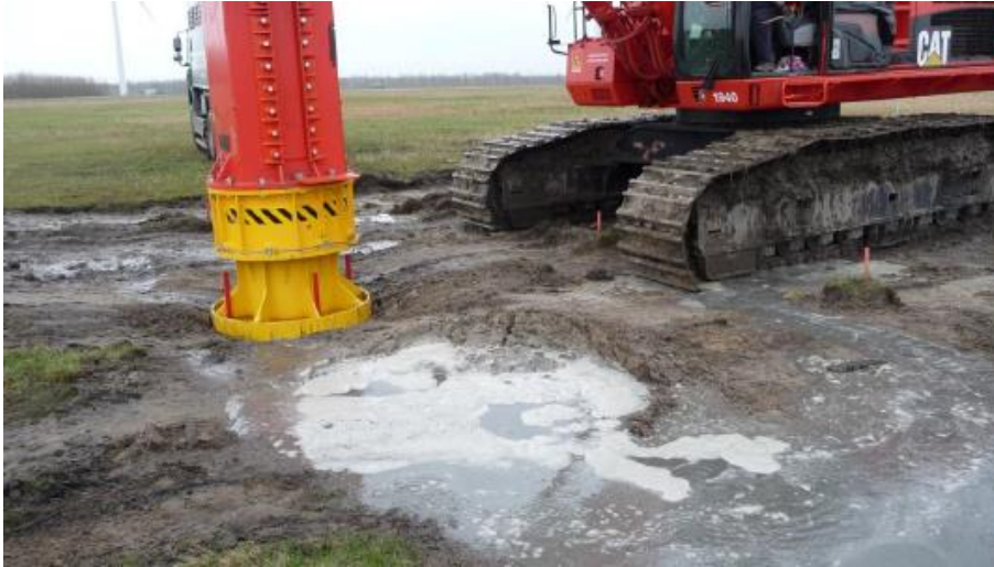
Figure 5-14: Flooding at the site due to the excess pore water pressure [13]
