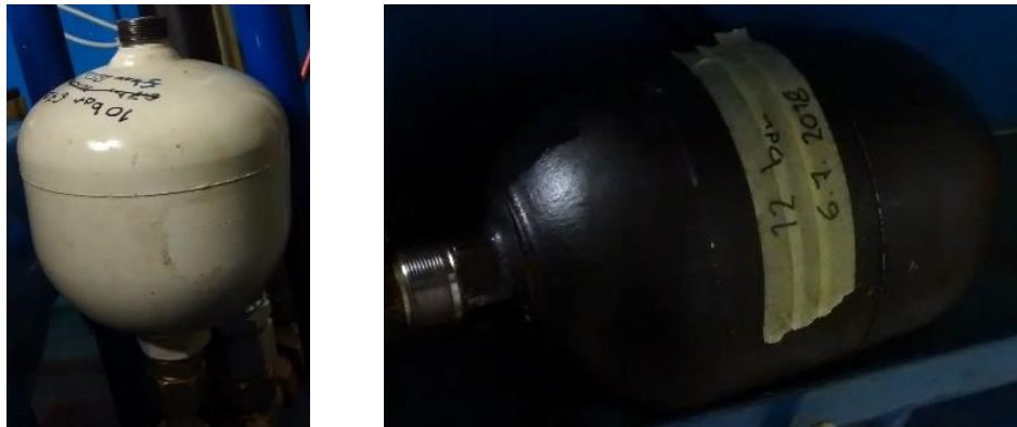
Figure 22. Low-pressure side accumulator (left) and High-pressure side accumulator (right)
