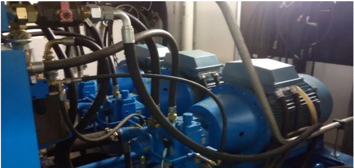
Figure 13. Main pumps for the hydraulic power source in the laboratory
