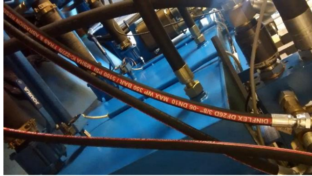
Figure 24. Flexible hoses in the setup
