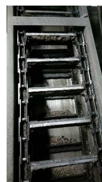
Figure 21 Sludge removal elevator, Suomenojan PP.
