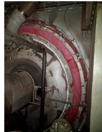
Figure 32 GT flue gas temperature measurement (wired sensors can be seen mounted radially on the outer rim), Suomenojan PP
