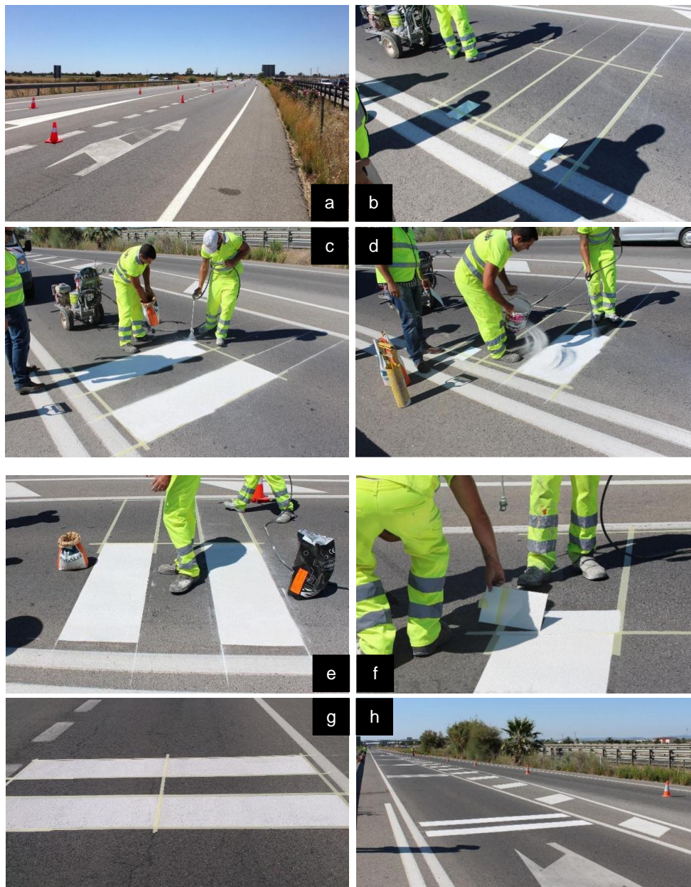
Figure 4. Sample fabrication process: (a) traffic diversion; (b) sample sketching with chalk and adhesive tape; (c) spraying of base material; (d) application of drop-on material; (e) in situ test sample finished; (f) laboratory specimen fabrication; (g) transversal stripe completed; (h) finished test section, ready to be opened to traffic.
