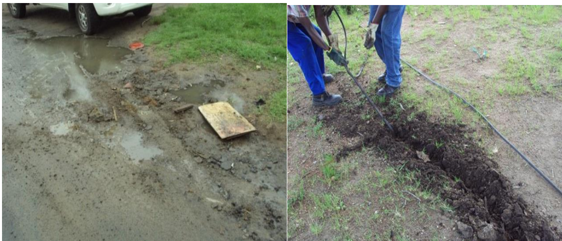
Photograph 3.7: Dangerous unauthorised electrical connections that were buried underground being disconnected and removed. 11
