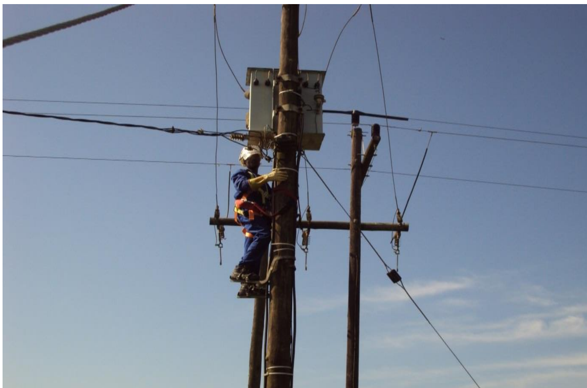
Photograph 3.10: ESKOM's removal contractor removing unauthorised electrical connections from an overloaded transformer in Jozini, KwaZulu-Natal, South Africa 14
