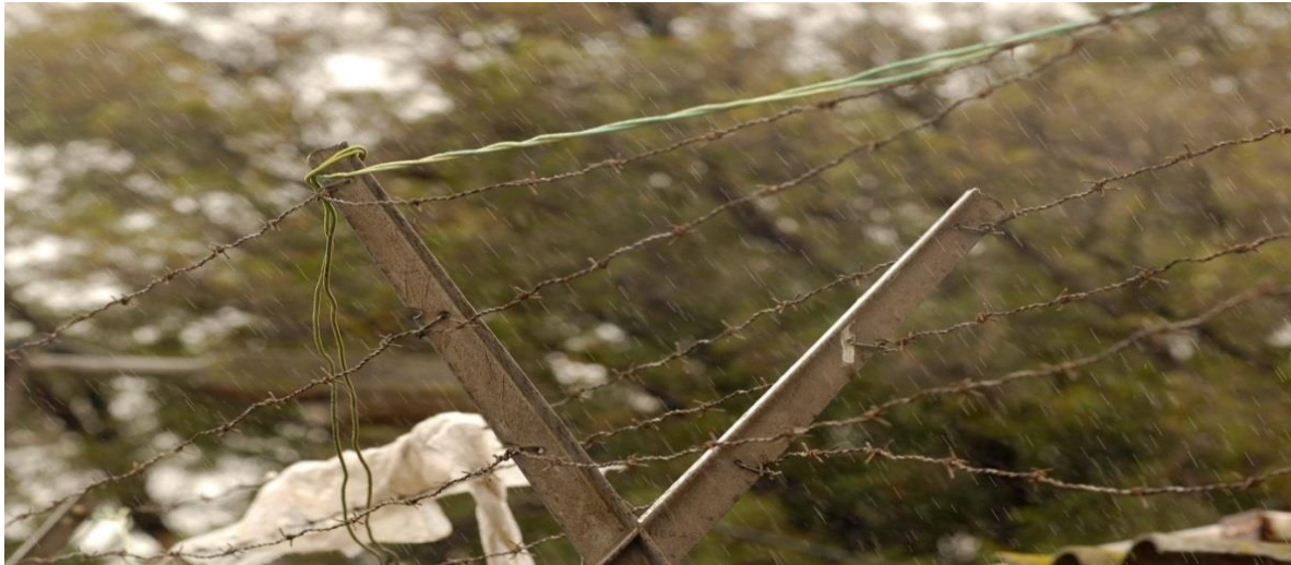
Photograph 3.3: Unauthorised electrical connections in Richards Bay, Empangeni, KwaZulu-Natal, South Africa 6
