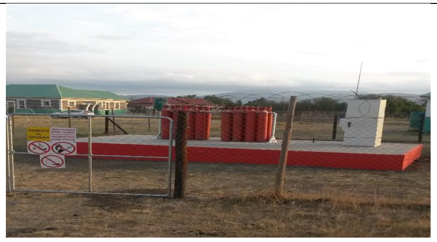
Photo 12: TECH4RED - School's hydrogen fuel cells for backup power
