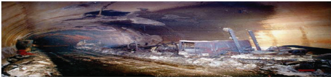
FIGURE 6. The fire damage to Mont-Blanc Tunnel [13]
