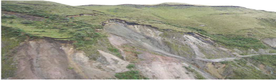
FIGURE 1. The landslide that affected the headrace tunnel [6]
