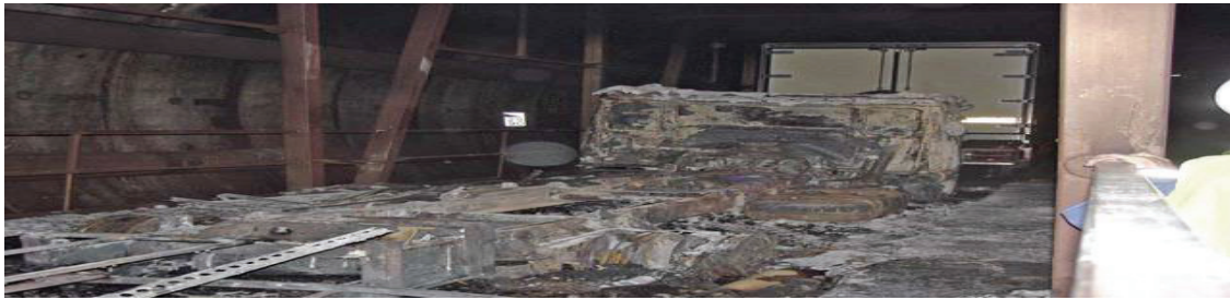
FIGURE 4. The fire damage to Channel Tunnel [10]
