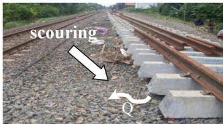
Fig.1. The scouring of rail ballast after flooding
