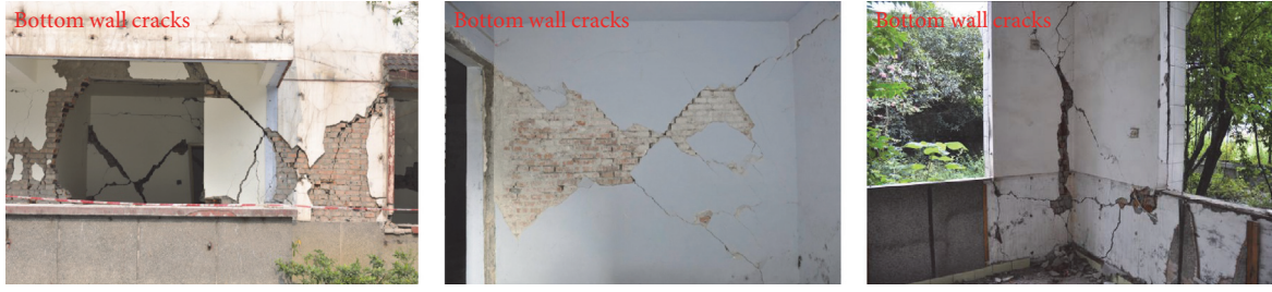
FIGURE 1: Damage of bottom masonry walls during the 2008 Wenchuan earthquake.
