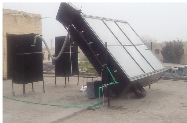
FIGURE 2. The flat plate solar collector assembly
