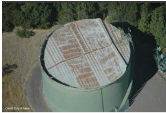
Figure 3-18 Napa Valley in 2014. Roof damage in Montana B tank
