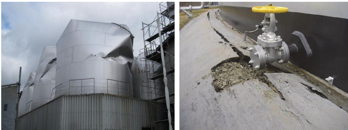
Figure 3-17 Tohoku earthquake in 2011. Silos damaged by ground shaking at Sendai harbor (a), tank settled because of liquefaction around the foundation
