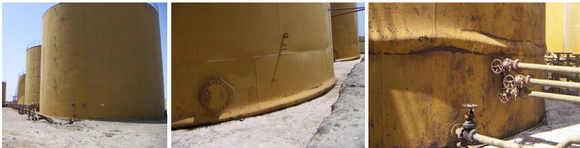
Figure 3-16 Central Peru earthquake in 2007. Blue Pacific oil facility view and tank damages
