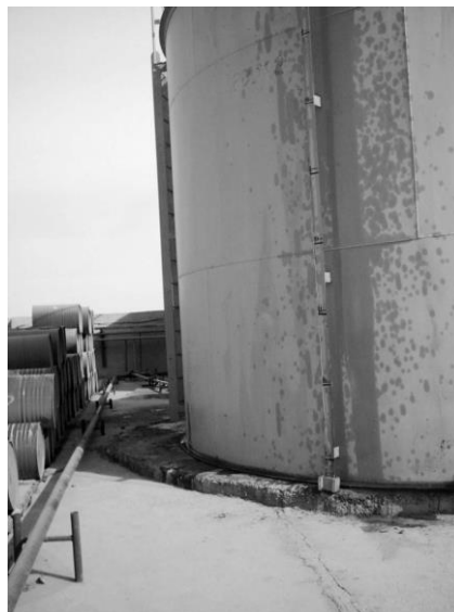
Figure 3-15 Bam earthquake in 2003. Leakage of oil from tank due to sloshing
