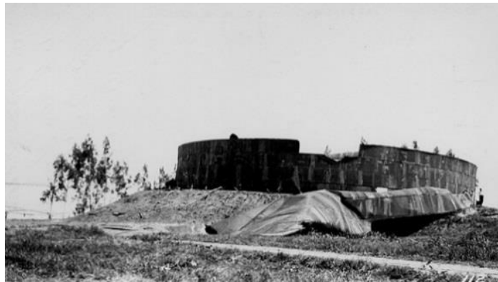
Figure 3-1. CLADWP Western Avenue riveted water tank, failure of the fourth shell course, Long Beach 1933
