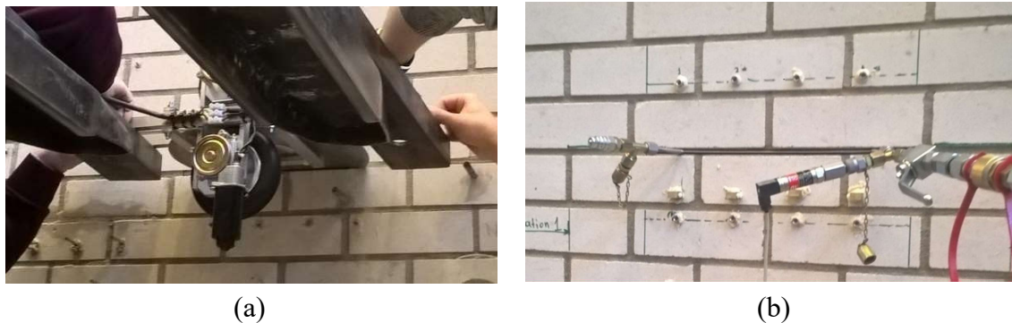
Figure 7.2. Case study – Single flatjack test: (a) execution of the cut; (b) seating of the flatjack.
