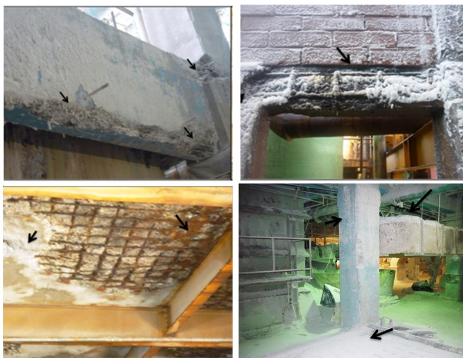
Fig. 2 - Structural elements deteriorated due to corrosion processes active during production.
