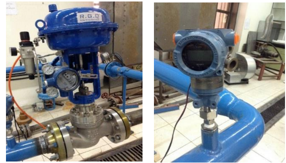
Figure 5- Valve installed in 3-in pipeline (left), Pressure transducers installed on pressure taps (right)
