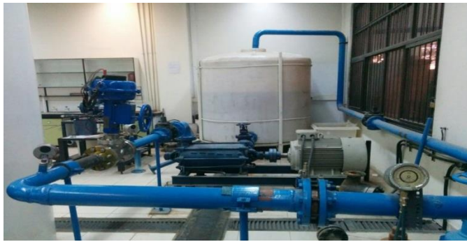
Figure 4- The test bench used for the experiment (Courtesy of Thermo-hydraulic Laboratory of the Iranian Ministry of Power)
