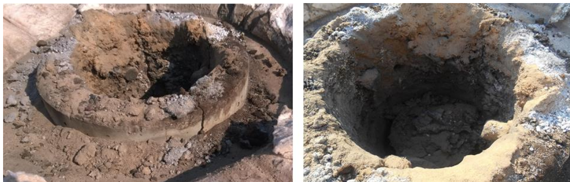
Fig. 2 Reactor lining with melted fuel parts and visible crack in lining
