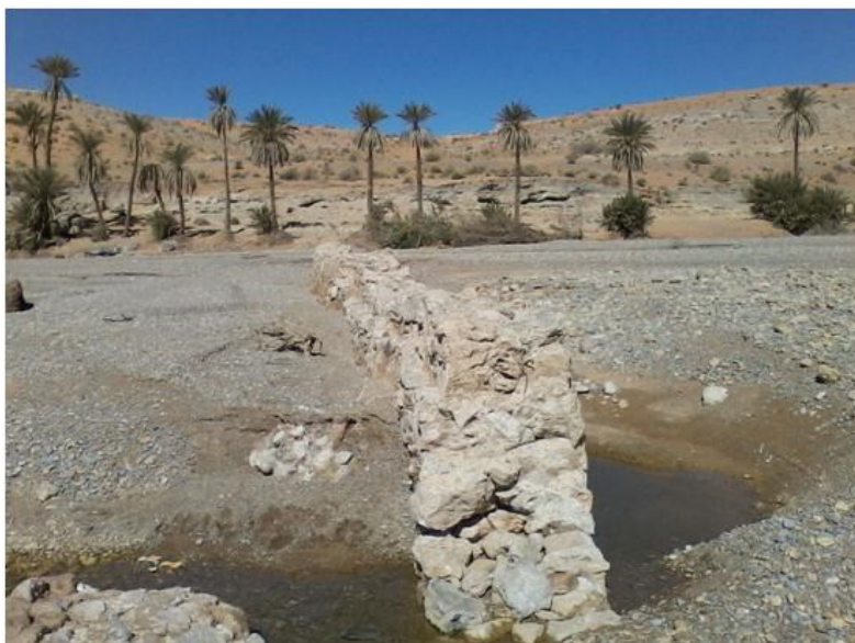
Fig. 5. Ancient dam destroyed by a flood (Photo. Authors, April 2015)
