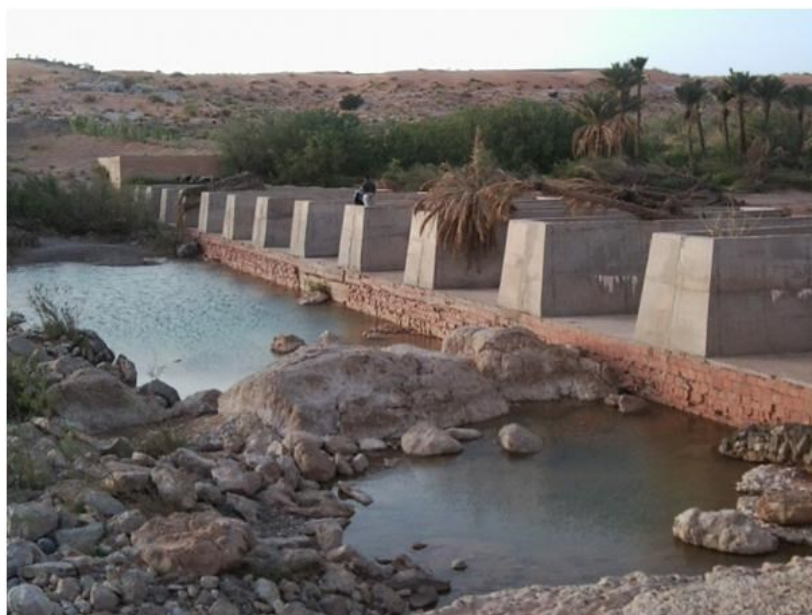
Fig. 6. New weir barrage constructed at the end of the years Ninety (Photo. Authors, April 2015)
