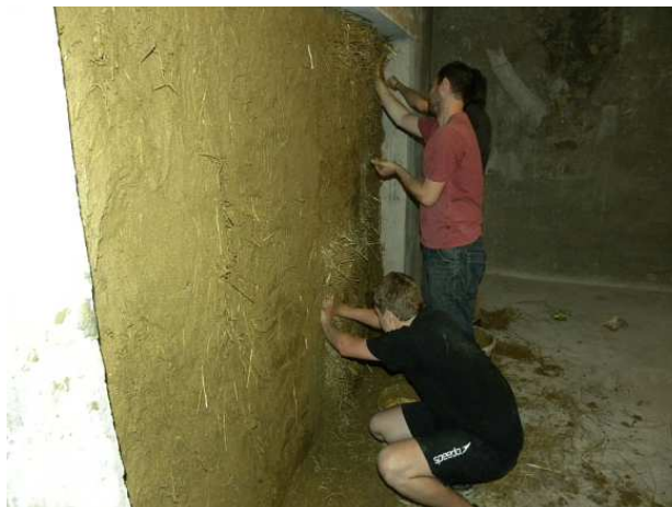
Fig. 4: Application of clay plaster on the straw bale wall surface. By author.
