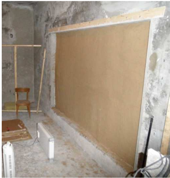
Fig. 9: View of the finished clay plaster on the interior side of the straw wall. By author.
