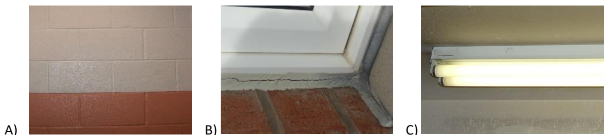
Figure 2: (A) Painted wall; (B) window caulking; (C) light ballast are all places where PCBs can be found in schools.
