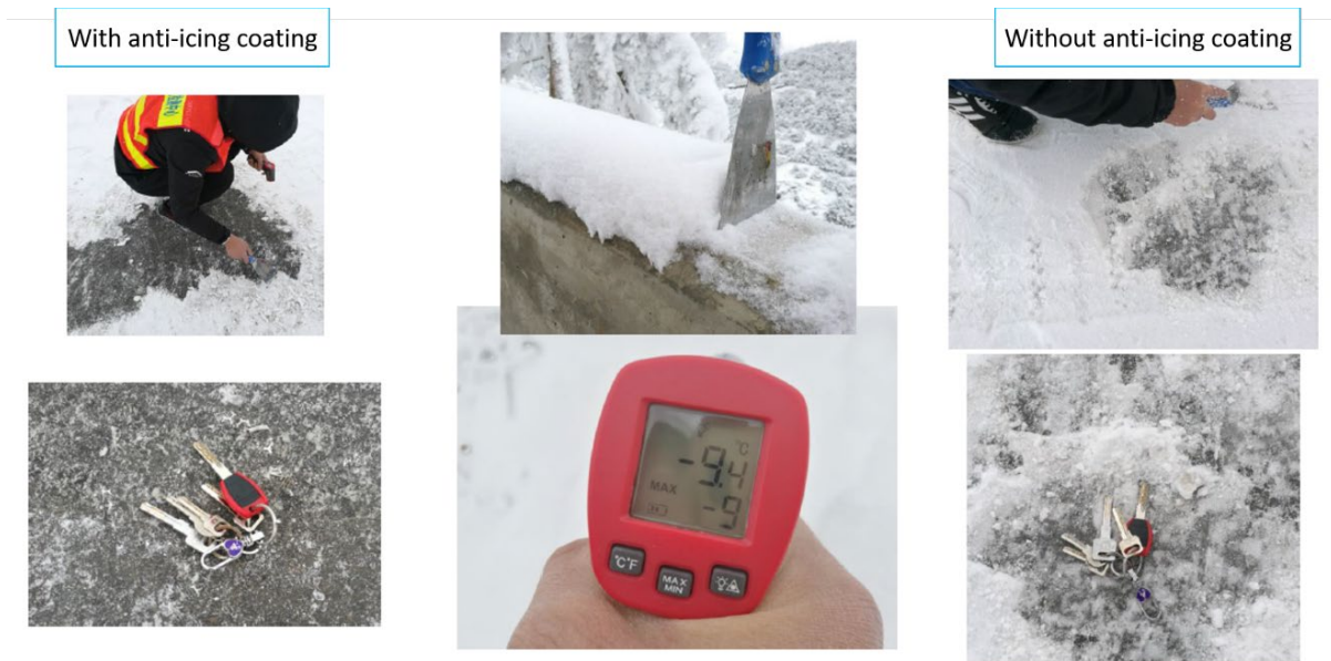
Figure 12. A section of the road in the Yunnan Province of China (it showed better anti-icing performance, with the snow thickness of 6 cm and the ambient temperature of -9°C).
