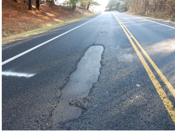
Figure 4. WinterPave failure Ohio DOT test sections on VIN-50 low-volume road tests (provided by ODOT, 2018, phone and email communication).
