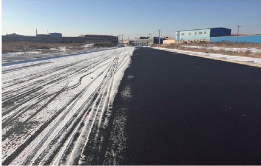
Figure 8. A section of the road in the Liaoning Province of China (-6 °C).
