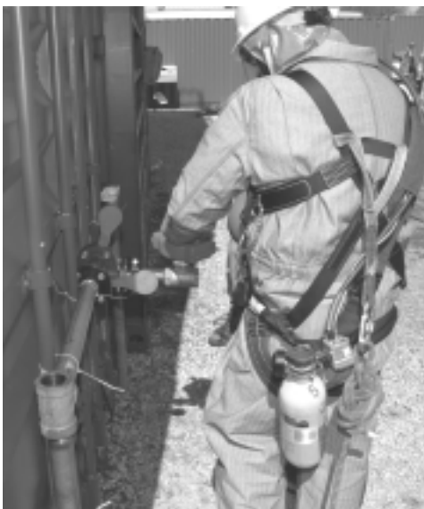
Confined Space Technician completing a double block and bleed to isolate the confined space prior to making entry.
