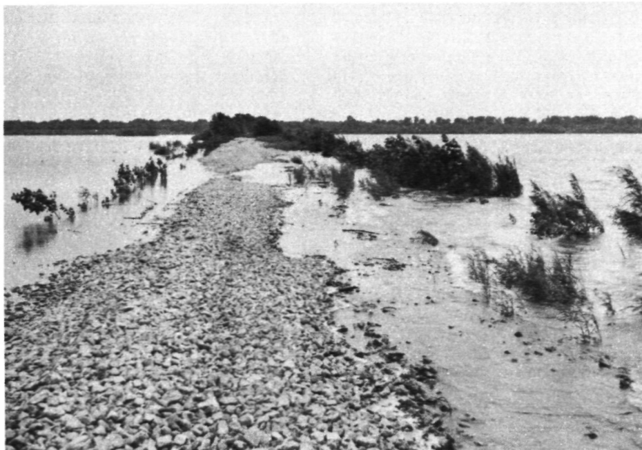
Figure 5. View Along the Top of the South Levee Looking Westward on July 20, 1950 Note flow into Lake Chautauqua from Quiver Lake (at left). Water level 439.1 Mean Sea Level
