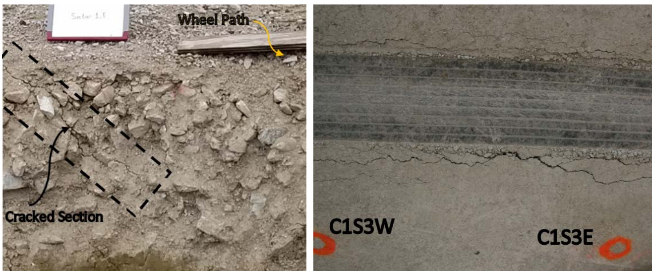
Cracking in C1S1E (PCR/QB1 – 2 Lifts)
