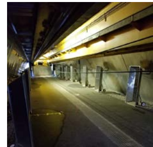
Heaters for Temp. Control
