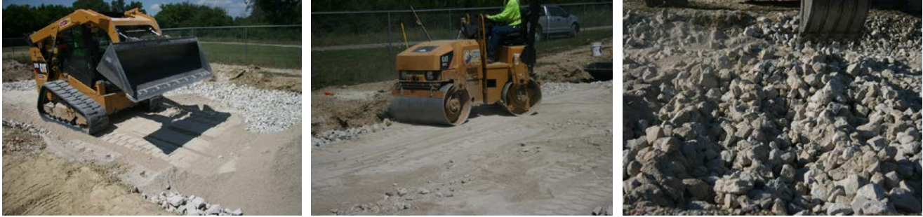
Construction of the first lift in the two-lift PCR/QB1 test section (C1S1)
