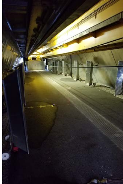
Heaters on Pavement
