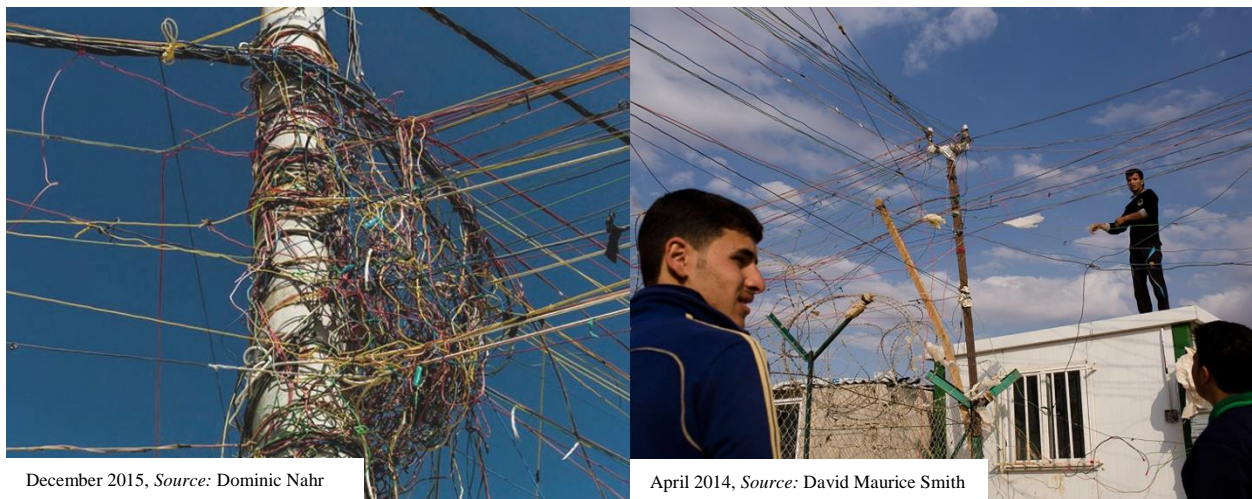
Figure 8: Drawing Electricity from al-Zaa'tari's Street Poles
