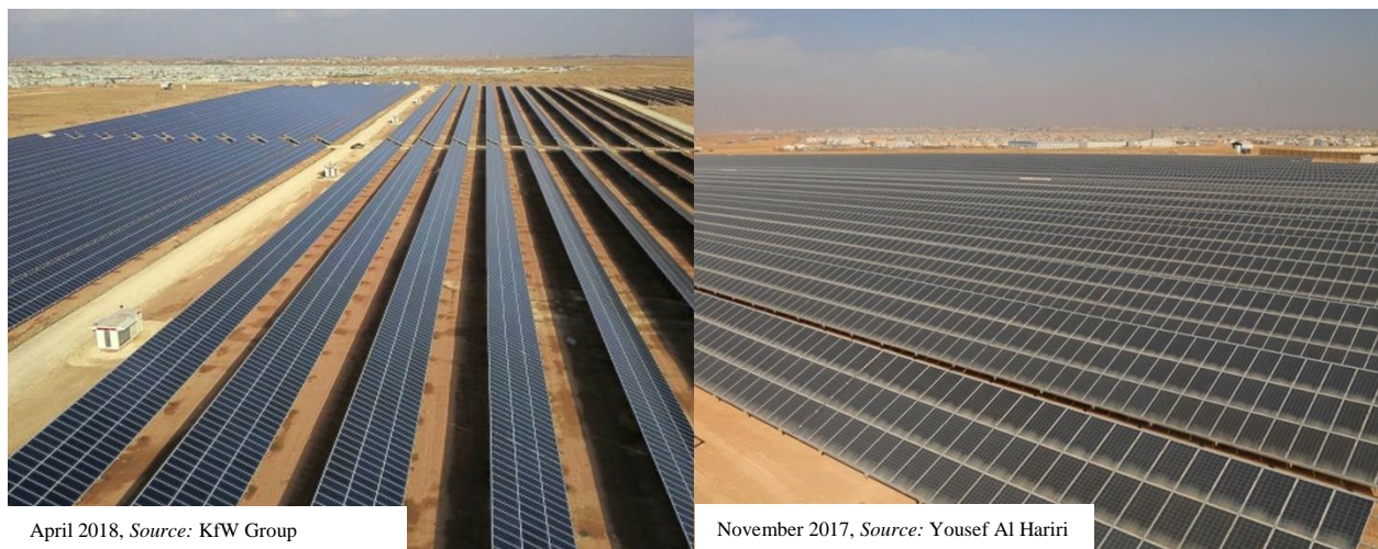
Figure 10: Al-Zaa'tari's Solar Power Plant
