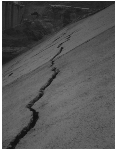
Figure 3.18: Crack occurred in cushion material of TSQ1 dam (Ma & Cao, 2007).
