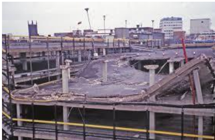
Figure 2.42. Pipers Row Car Park, Wolverhampton Partial Collapse, March 1997[143]
