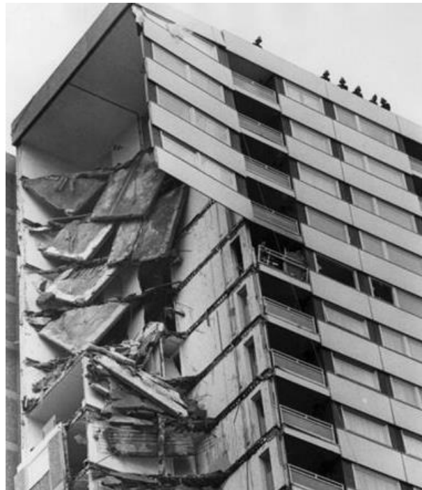
Figure 2.1. Ronan Point after the domestic gas explosion 1968 [6]
