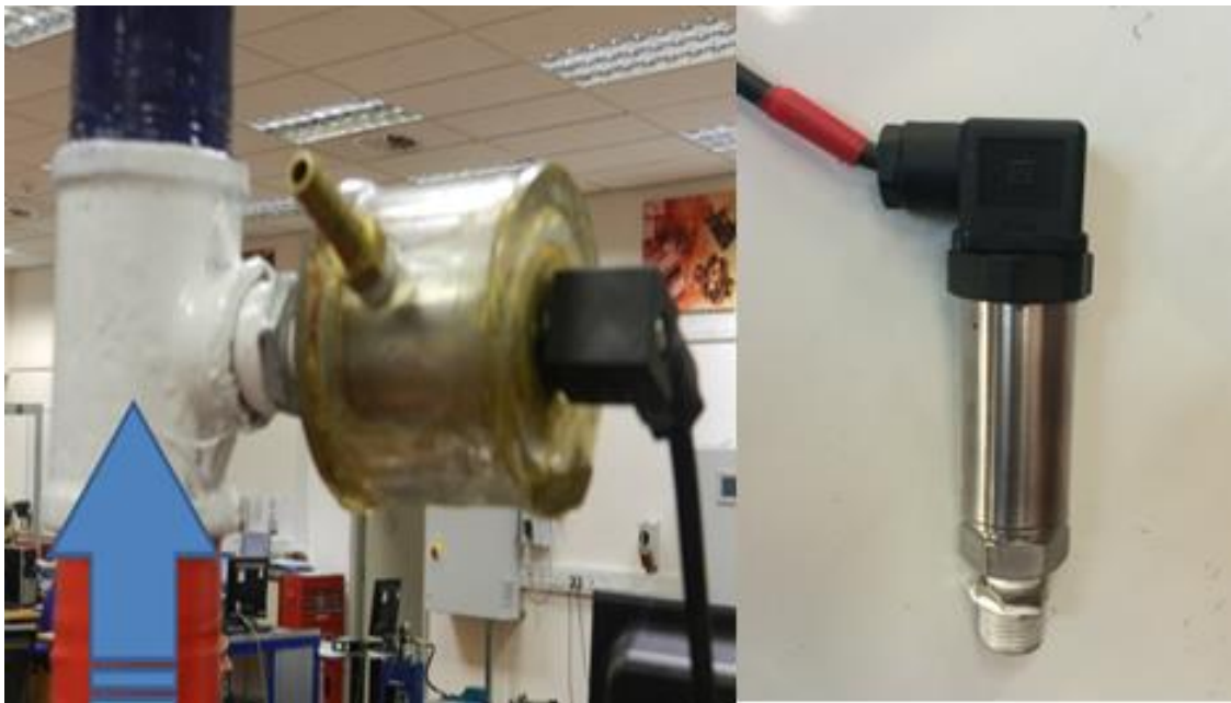
Figure 5-6 Pressure transducer in discharge line at the pump outlet
