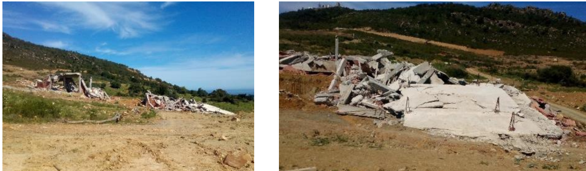
Figure 6.9: Destroyed illegal constructions in Amezoui, jijel.
