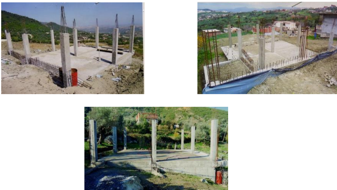
Figure 3.8: Completed work for the application of the second instalment, December 2016 (Source: Housing department)
