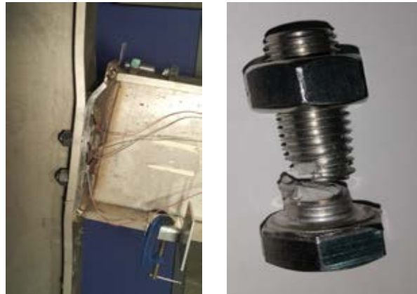
(a) Flush End Plate (FEP-O) connection failure mode and fractured top bolt
