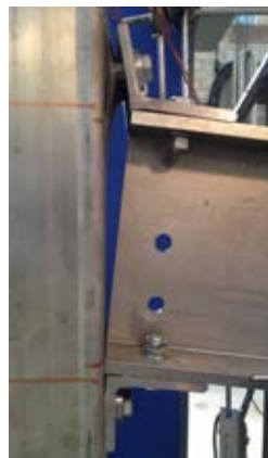
(b) TSAC-T-2: deformation of angle cleat, column face and sleeve Hollo-bolt
