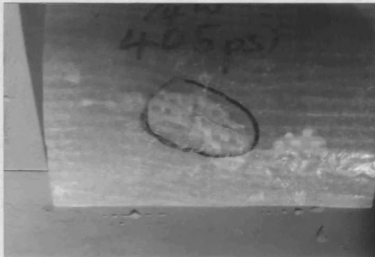
Region of poor reinforcement alignment.
