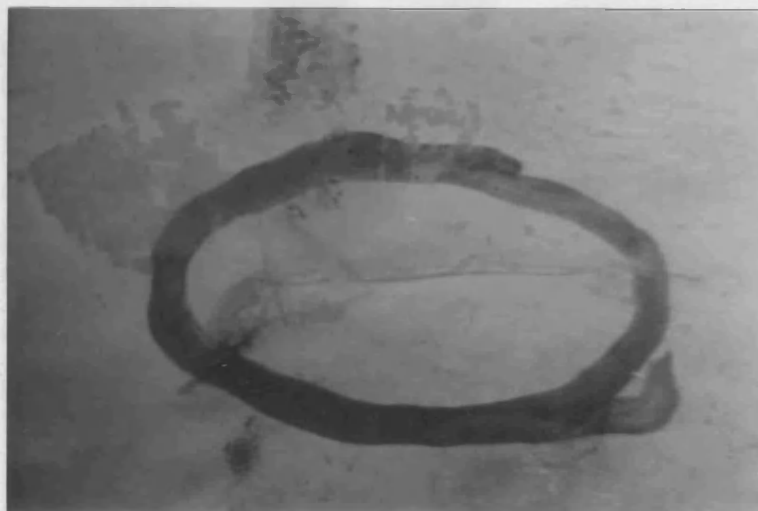
Point of leakage in a failed virgin pipe.
