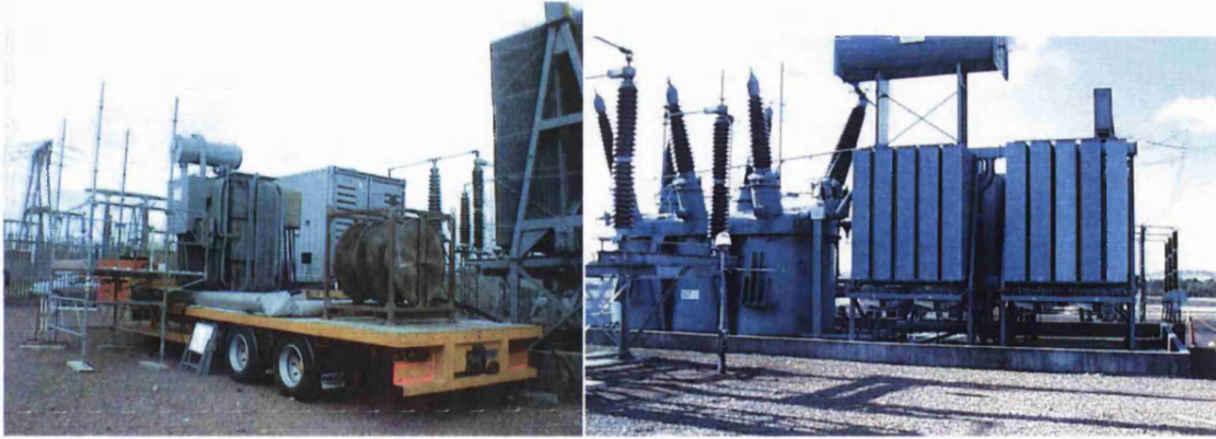
Figure 6.1: A diesel generator unit and a step up transformer 0.433/33 kV (left) and a 400/275/33 kV transformer (right) under test for PD-diagnosis
