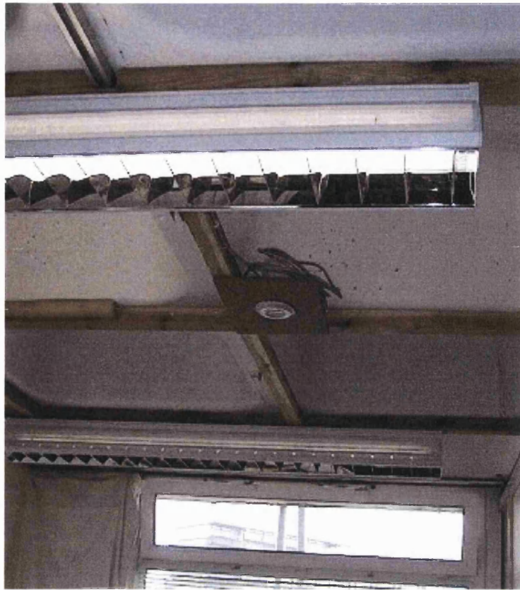
Figure 6.10: Picture showing the rear light brighter than the window light for daylight linking.
