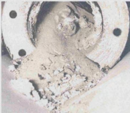
Figure 4.119 Run 9:Combustion Tube at Ignitor
