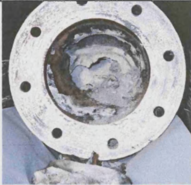
Figure 4.87 Run 6: Combustion Tube at Ignitor
