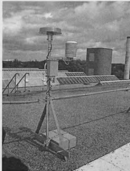
Figure 3. 2 GPS receiver and attached meteorological sensors
