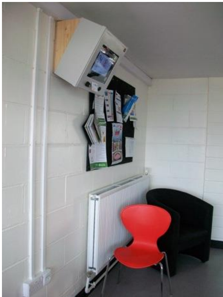
Figure 5.1. Tablet installation setup
