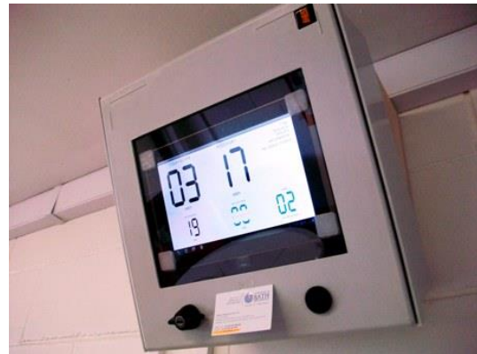
Figure 5.2. Tablet affixed to cabinet
