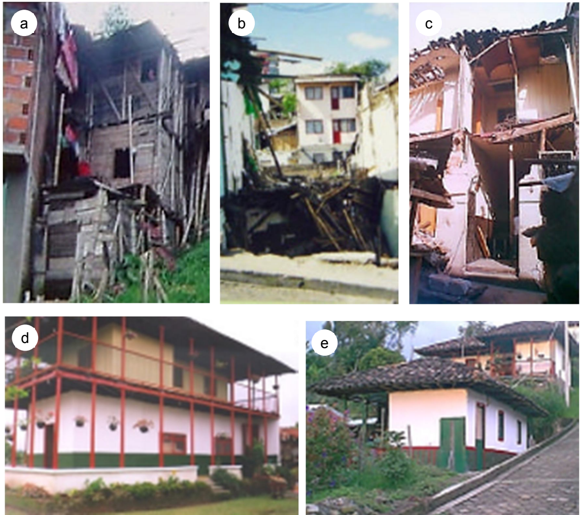
Figure 3-14. Construction with Guadua prior and post the 1999 earthquake in the coffee region, Colombia (Gomez-Buitrago, 2002). a) Shanty-town building. b) Collapse of a Guadua building due to unstable soil. c) Collapse due to discontinuity and inadequate combination of materials. d) & e) Houses that did not suffer collapse thanks to the correct use of building techniques with Guadua.
