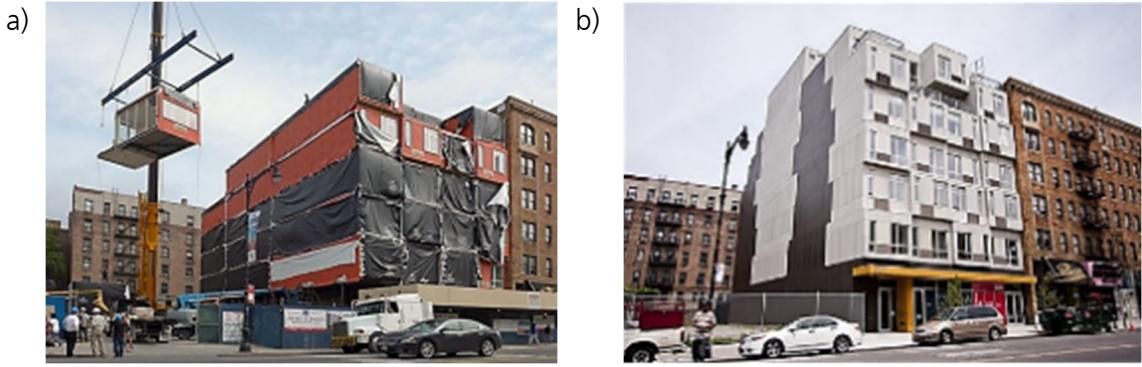
Figure 11-8. The Stack in New York city, a prefabricated seven-story by Gluck+ architects. a) Crane assembly of the volumetric prefabricated unit ( www.savemarinwood.org ). b) Finished building ( www.jcsa.com ).
