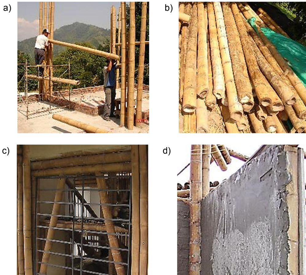
Figure 3-15. Some common issues in construction with Guadua. a) Intensive labour. b) Material irregularity. c) Incompatibility with building elements. d) Thick cement renders that generate a high environmental impact.
