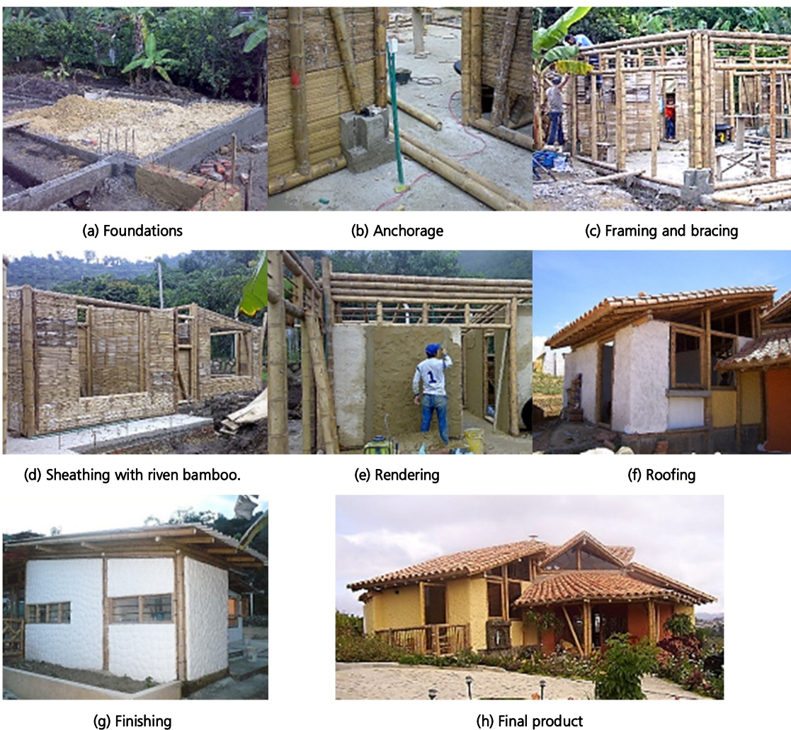
Figure 3-10. Construction process of the plastered cane wall framing system (picture (h) by Arme Ideas en Guadua Ltd).
