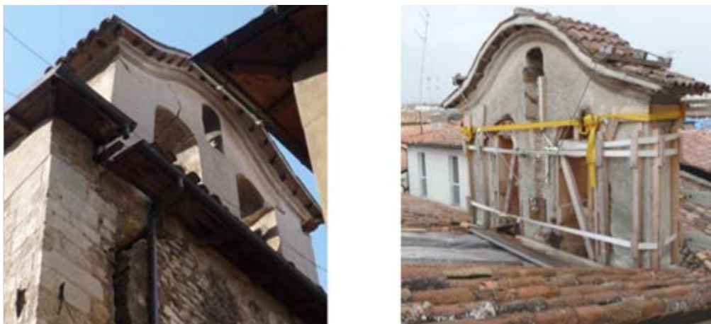
Fig. 5-8: Damage to the belfry (D9.1, NIKER project)
