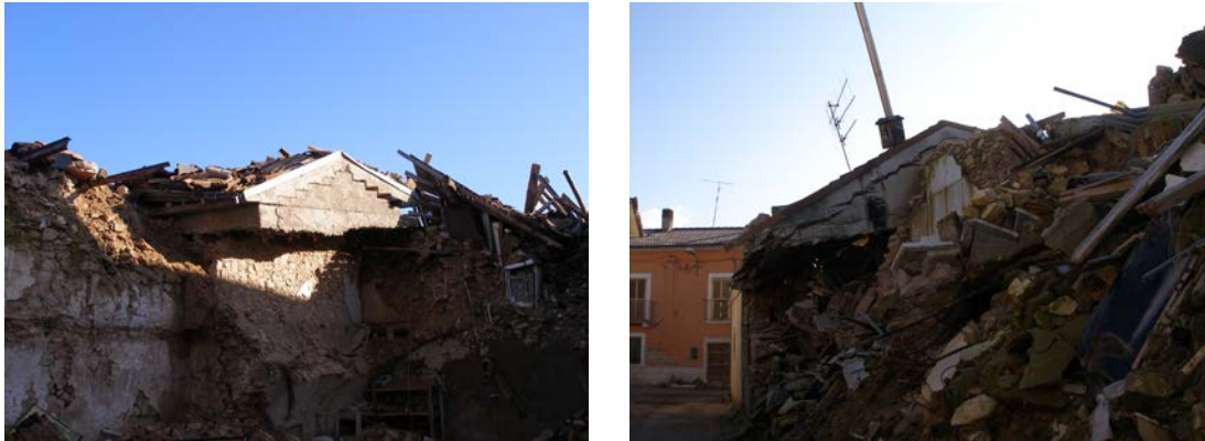
Fig. 2-1: Examples of collapses due to r.c. ring beam/ roof structures at top level of masonry buildings. Onna, L'Aquila, Italy, January 2010 – Eight months after L'Aquila earthquake, 2009. Author's own
