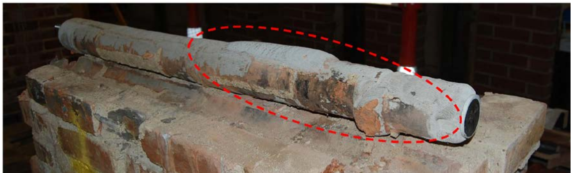
Fig. 4-27: Irregularities of grouted sleeve causing mechanical locking
