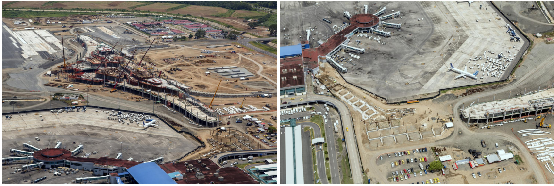
Figure 4-11: Tocumen airport extension on site, with link bridge foundations and columns being constructed. Source Foster + Partners.
