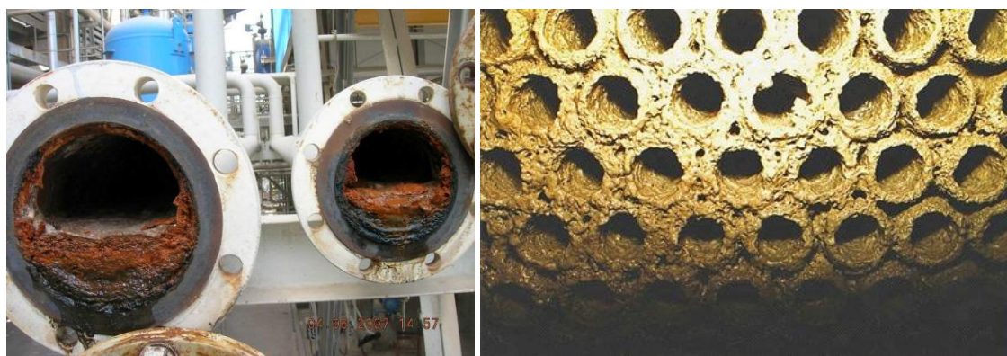
Figure 1: a) Microbially-influenced corrosion inside an oil refinery pipeline (MERUS 2011). b) Biofouling inside a condenser tube (Daniels and Selby 2007)
